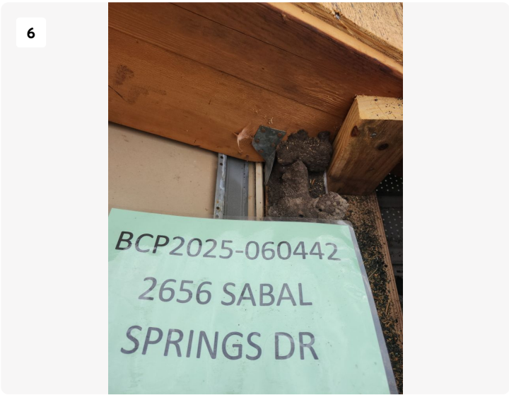
Project: 2656 Sabal Springs Dr Date: Jun 19, 2025, 9:06 AM Creator: Lucio Roofer
